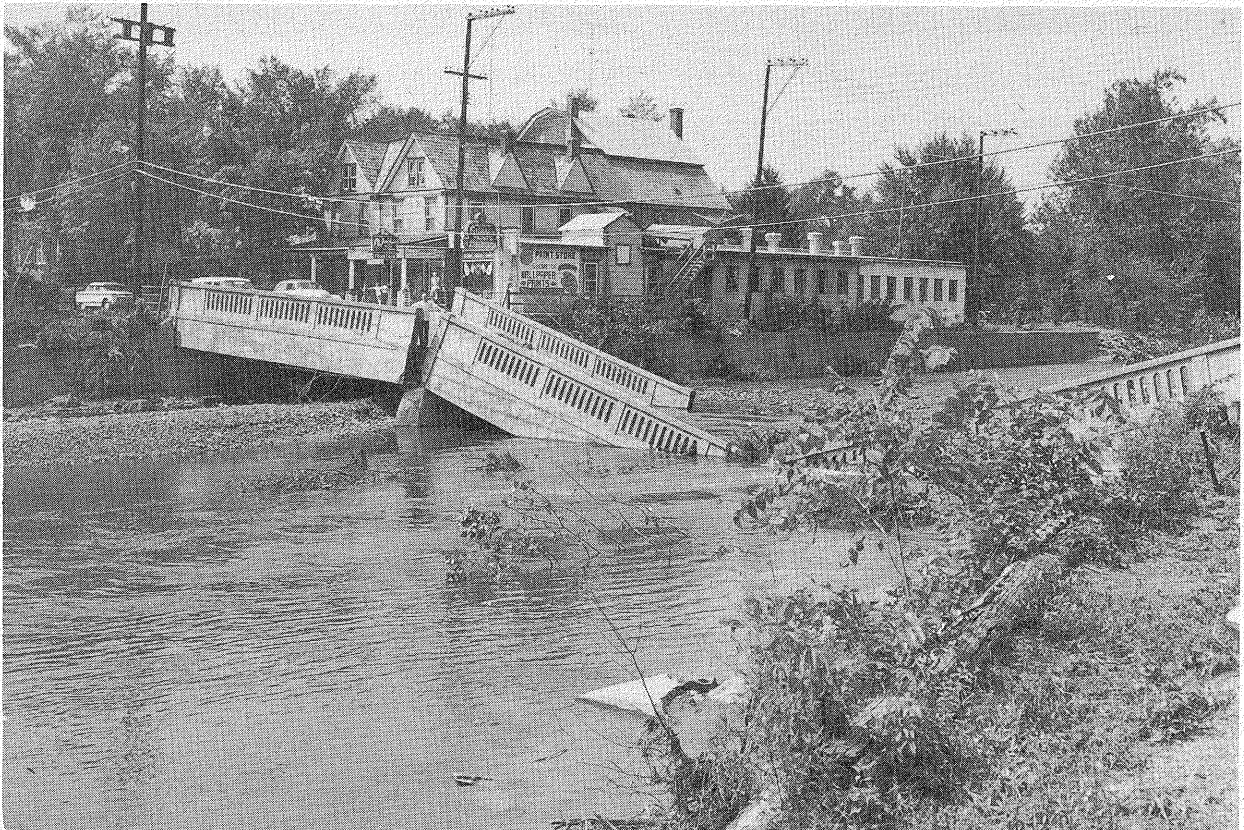
PLATE 7B.—Damaged bridge on Main Street, Stroudsburg, Pa. (Photo courtesy Pennsylvania Department of Highways.)
