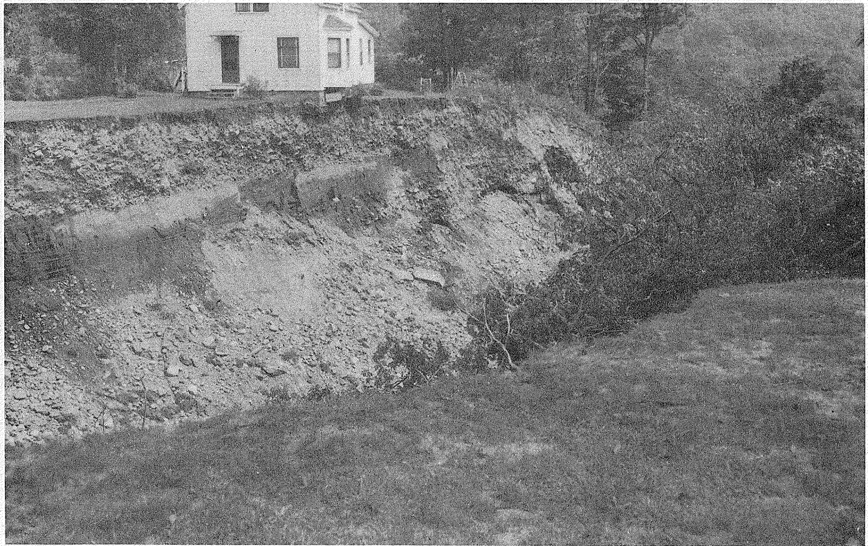
PLATE 6B.—Russell, Mass. Washout where no stream previously existed.
