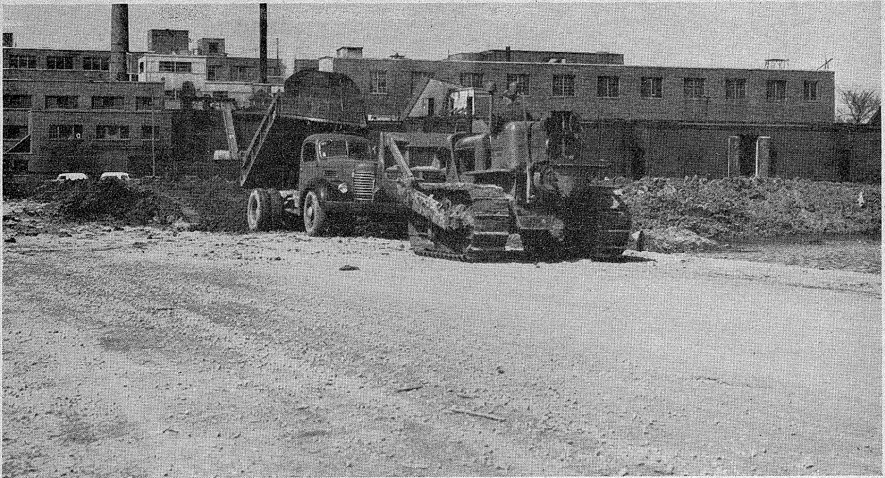
A. Dubuque, Iowa, April 17, 1952. Construction of dike around Dubuque Packing Co. 8 days before crest. (Courtesy Mel Schieltz, Telegraph Herald.)
