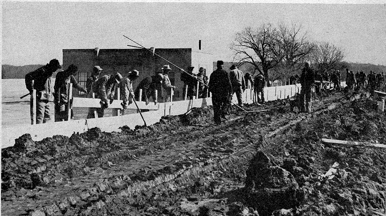
B. Flashboards going up at waterworks north of Council Bluffs, Iowa, days in advance of the crest. These were reinforced by sandbags, front and back. About 800,000 board feet of lumber were used. (Courtesy Omaha World Herald.)
